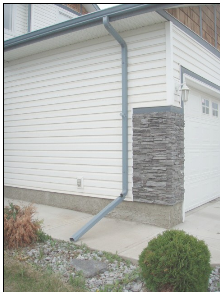
TYPICAL TRIP HAZARD
